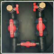
House connection chamber
